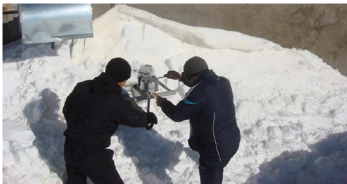
Ara Babayan and Karen Asatryan repairing the electric field meter on the roof of one of the buildings (completely under snow) at the Mt. Aragats Research station, 10,500 ft. elevation.
